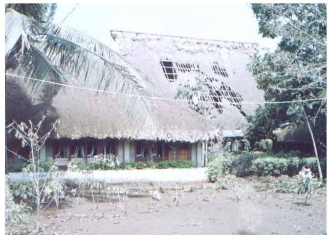
The ash-damaged roof of the school.
